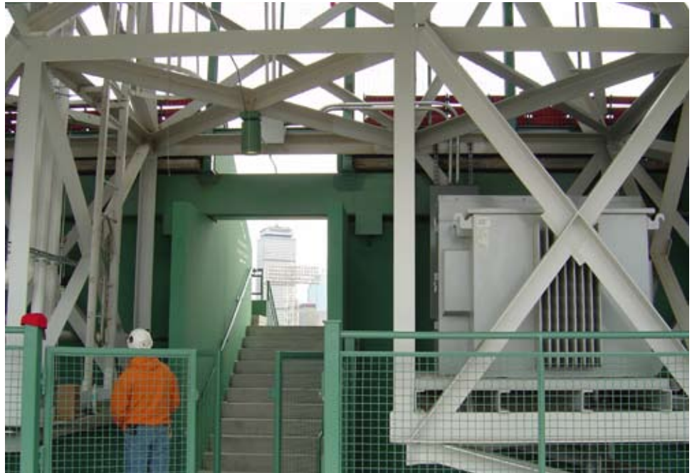
An FR3 Fluid-filled transformer is integrated into Fenway Park’s structure.
