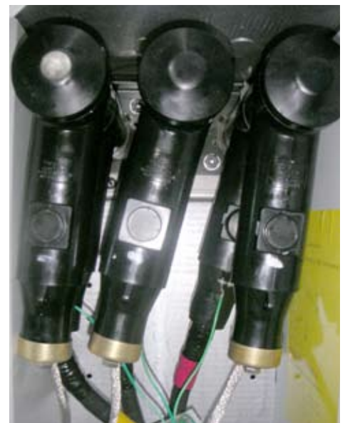
The new 17 kV arrester is used to protect the switchgear and the system from damaging overvoltages.
