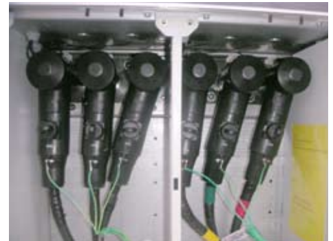
Typical application in RMU switchgear.
