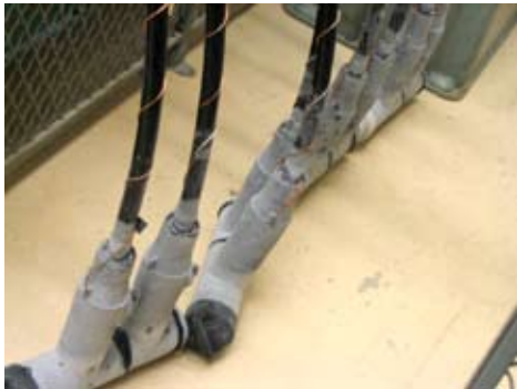
Connectors after testing.
