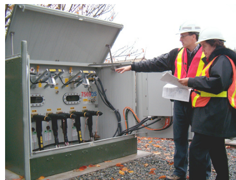
Russ Dobie (Project Manager) and Helen Iosfin (Distribution Planning Manager) inspect a Loop Tap Switch.
