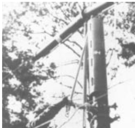
Figure 30. Pole cover prevents accidental contact of energized wire with pole while men install line guards to protect them from conductors.
