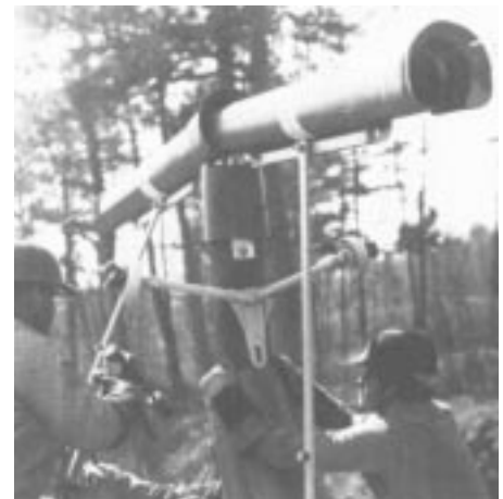
Figure 8. Line guards and pole covers increase safety as linemen install armor rods.
