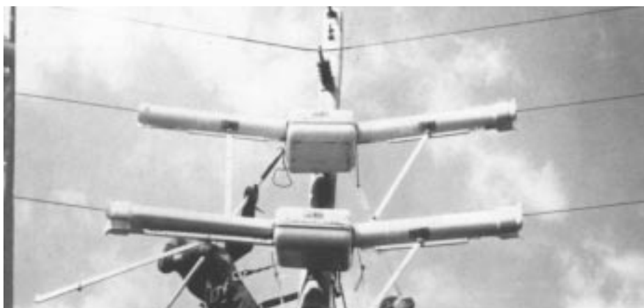
Figure 16. Line guards and insulator covers are installed to assure safety during work on pole with stand-off insulators at point where there is a small angle in the line.
