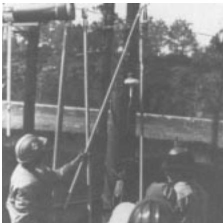
Figure 17. Line guards shield against contact with conductor while armor rods are installed.
