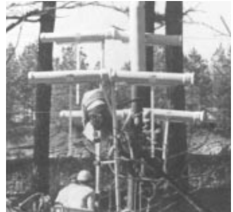
Figure 7. Crew assures safety by installing line guards and pole covers while working on 12 kV line with armless construction. Insulator covers, yet to be installed, will complete protection.
