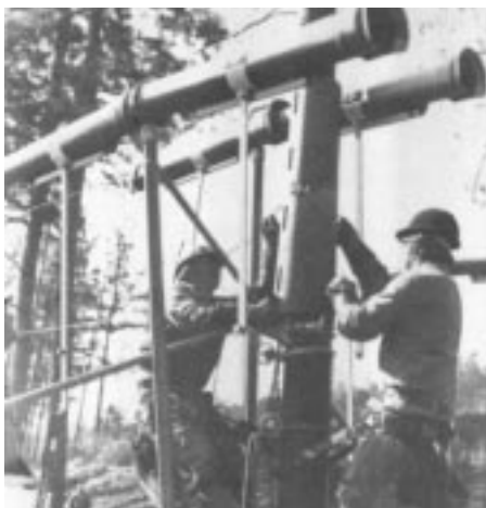
Figure 22. With wires held off with hot sticks and line guards in place, pole cover is installed to prevent energized wire from making contact with pole.
