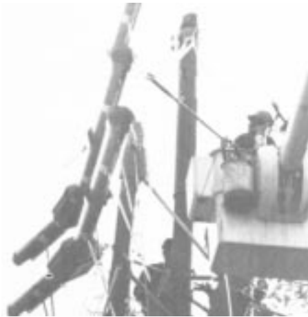
Figure 10. Line guards, stand-off insulator covers and pole covers installed on angle pole with strain insulator construction assure safety while conductors are transferred to new pole at right.
