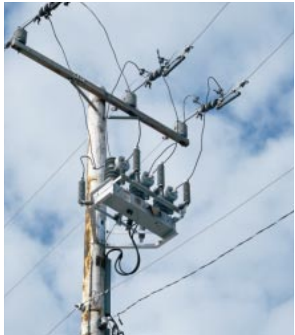
Installed Kyle NOVA three-phase recloser.
