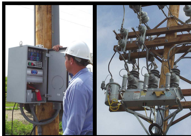
Jim Cook, Electrical Engineer, Woodruff Electric with Form 6 control. Installed NOVA™ recloser.
