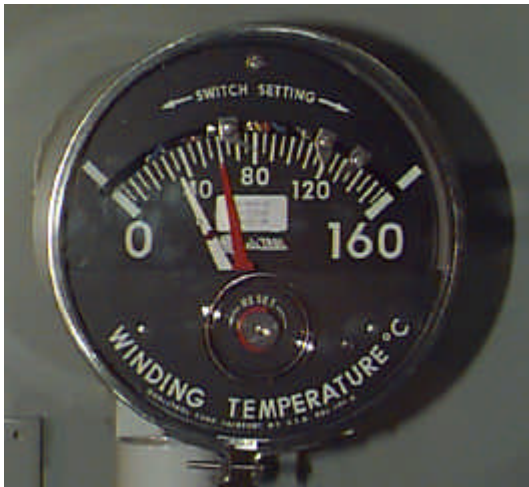
Figure 7. Winding Temperature Gauge
