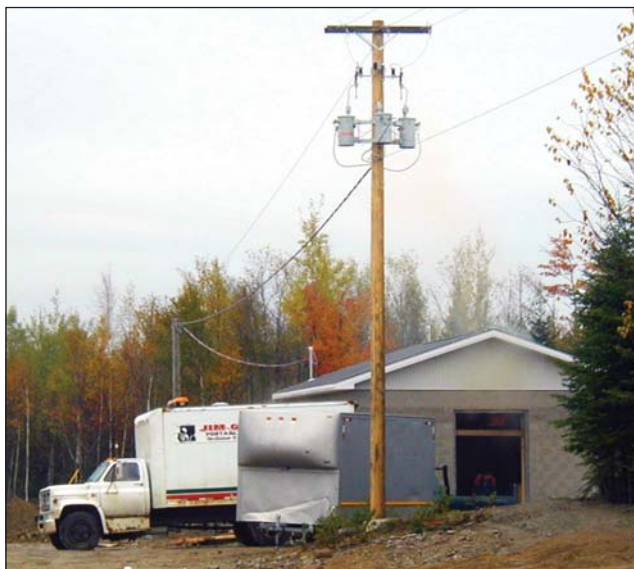
McAdam wellfield pumphouse and transformers filled with Envirotemp FR3 fluid.
