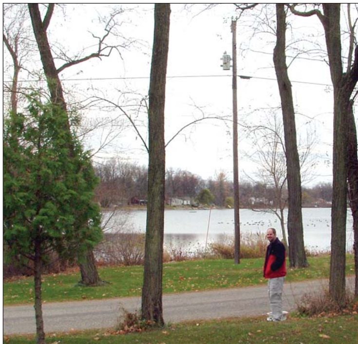
Jamie Shields (Steuben County REMC) at Wall Lake with Cooper Power Systems Envirotran pole-mounted transformers filled with Envirotemp FR3 Fluid.
